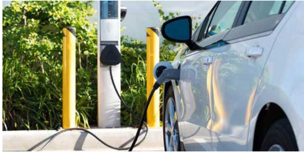
Figure 105: Public carpark electric vehicle charging station, Washington Source: www.greenlight-solar.com
